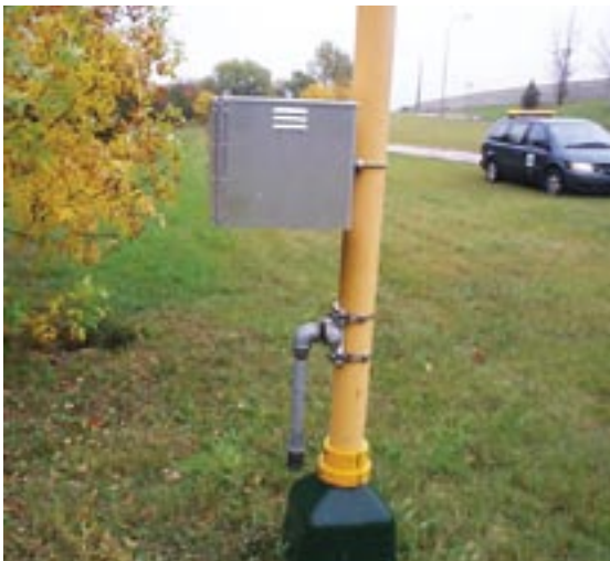
Sensor inside galvanized pipe
